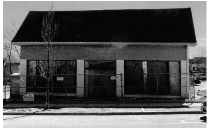
The building (pictured during the renovation process) was in dire need of restoration.
